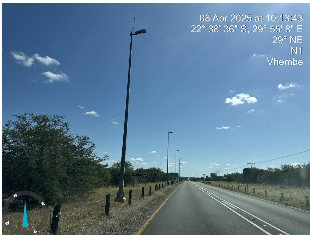
Photo 7.35: Lighting infrastructure along the N1 national route
